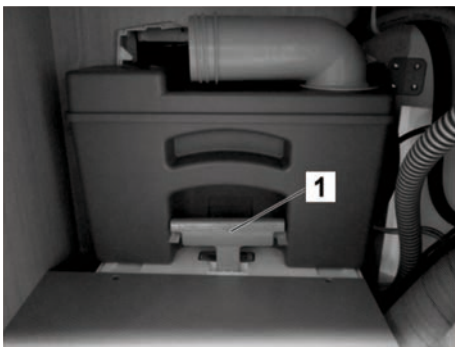
Fig. 179: Waste holding tank in the disposal shaft
